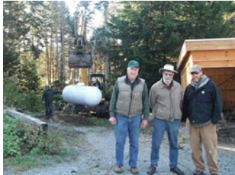
Phil Whitney, Chris Johnston, and contractor Jesse Jameson on site for Groundbreaking Day.
