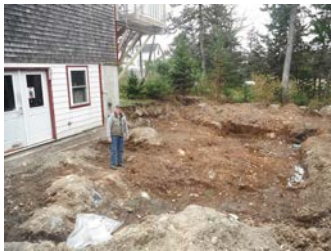
Earthwork and foundation construction began in October in order to be completed prior to freezing weather and to minimize disruption to Cranberry House operations in the summer of 2019. The foundation is 20' x 30' and will support an expansion of all three floors.
